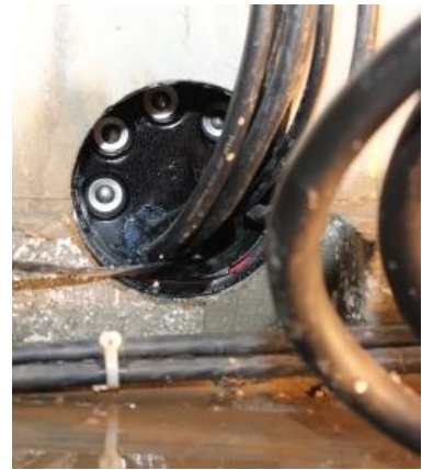
Photo: Water ingress in a power station at the Altenburg-Nobitz solar park
