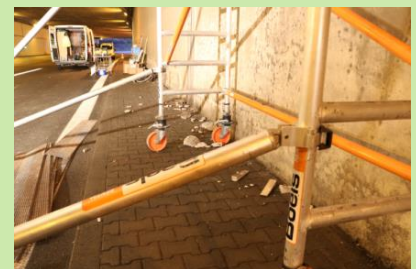
Concrete debris, formwork timber and nails
