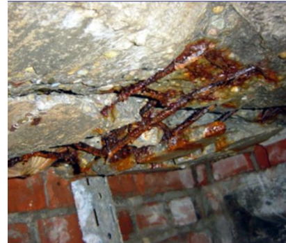
The bridge deck has cracked
